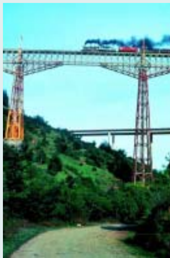
The Malleco Viaduct (in La Araucanía). Inaugurated in 1890, it is one of Chile's most outstanding examples of metal engineering. Its frame was constructed in France from 1886 to 1888, and it is 347. It is 2 meters long and 102 meters high.
